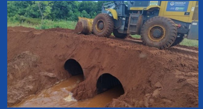
Donation of HDPE pipes for maintenance of a bridge providing access to rural residents, in partnership with the Municipality of Inocência.
